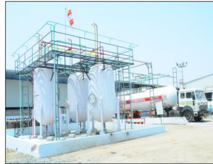
Anhydrous Ammonia Unloading & Storage
